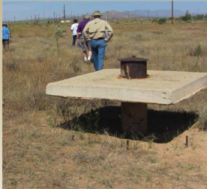
Subsidence, leaving Well head exposed above ground
