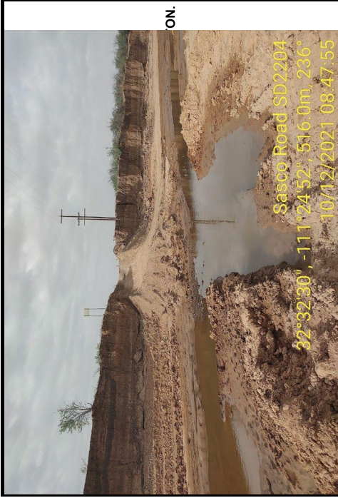
Sasco Road Damage, 10/12/2021 Photo By DEMA
