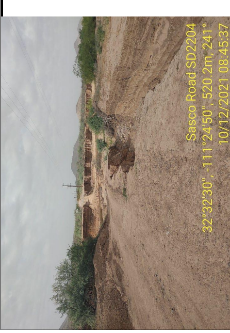
Sasco Road Damage, 10/12/2021 Photo By DEMA
